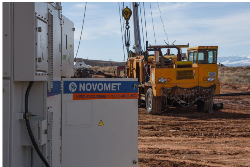
When the first ESP permanent magnet motors used in the Big Horn Basin were installed in gas-plagued wells, the operator was testing efficiency. What it got in return was an increase in ESP runlife of over 800%.
